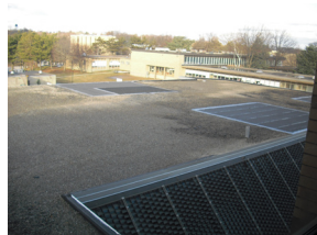
Priority 3 Example Correct ponding issues on roof
