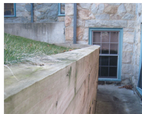
Priority 2 Example Repair retaining wall
