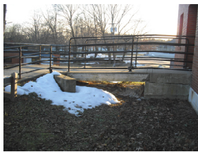
Priority 1 Example Replace deteriorated handicap ramp
