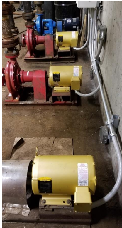
Horace Mann New Energy Efficient Motors
