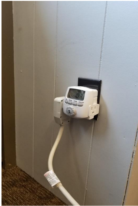
Physical Plant New Window AC Timer
